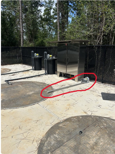
Typical installation: blower (circled) on the slab beside the control panel, with a stainless air line into the wet well hatch.
